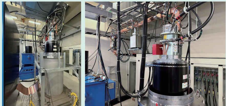
Fig. 7: Installed K1 Station (left) and RF transmission line (right).
